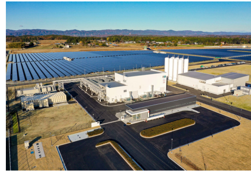
Following the Great East Japan Earthquake in 2011, Namie Town has focused on introducing renewable energy and hydrogen in an attempt to rebuild better. In 2020, the New Energy and Industrial Technology Development Organization (NEDO) began hydrogen production demonstrations at the Fukushima Hydrogen Energy Research Field (FH2R). TOSHIBA ENERGY SYSTEMS & SOLUTIONS CORPORATION
