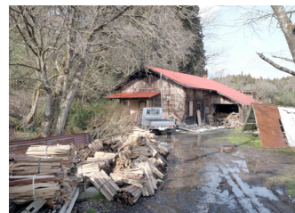
Shinohara's workshop in the mountainous area of Suzu. The brick-built kiln inside the workshop completely collapsed during the January 1 quake, with firewood scattered everywhere.
