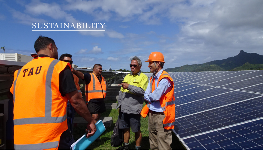
Left: Staff inspect a photovoltaic power generation facility in the Cook Islands. Solar power is an efficient way to generate electricity for the countries of Oceania located near the equator.
